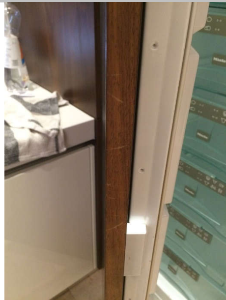
Edge of door freezer cabinet
