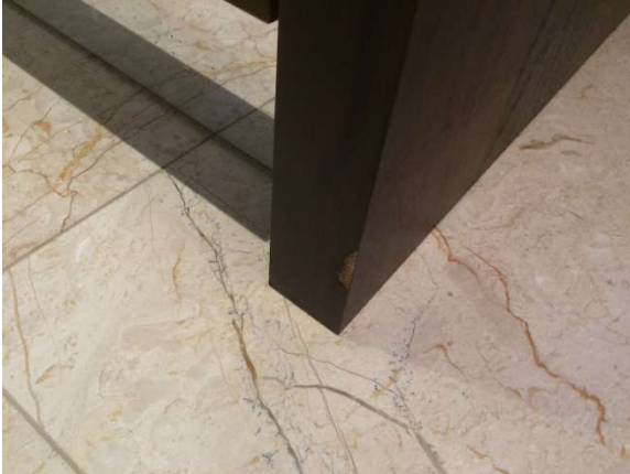
Bottom right panel fridge cabinet
